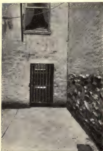
FIG. 105.—A portion of the bottom of a new-law court, showing tunnel for circulation of air.
